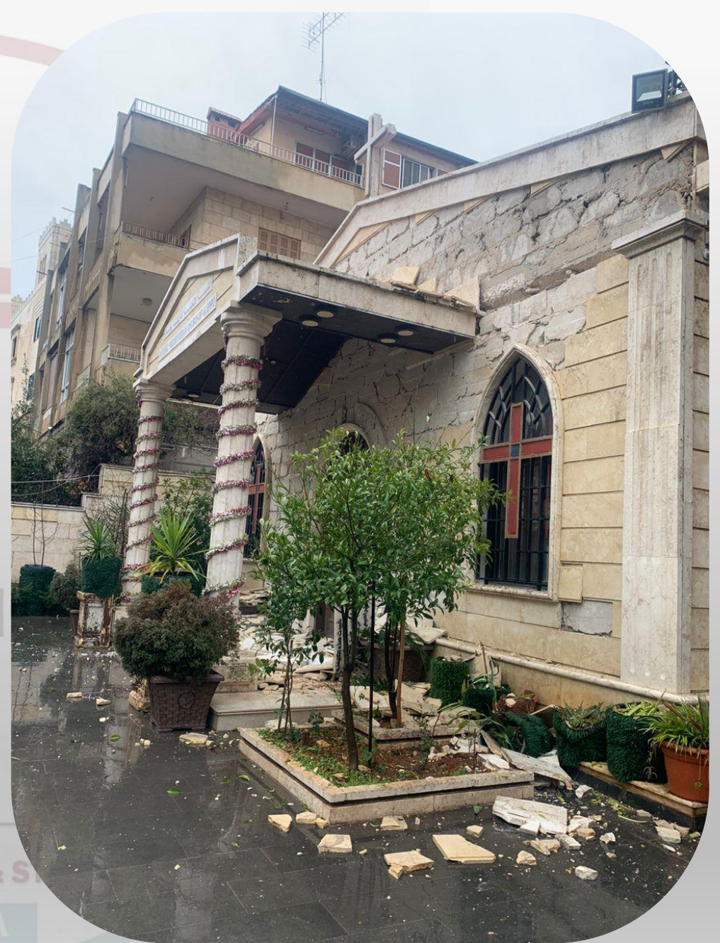
The Church Facade after the earthquake
